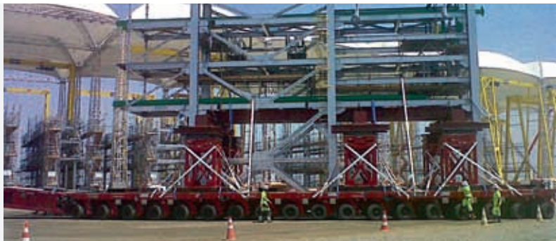
A pipe rack for the COMPERJ refinery project. Photograph courtesy of Petrobras and CPPR.
