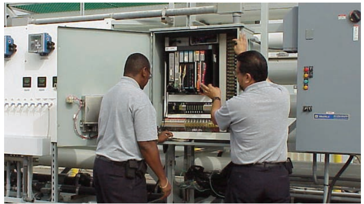
Photographs courtesy of Long Beach Water Department.
