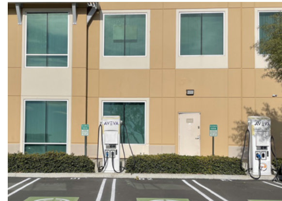
EV charging at our Lake Forest, California offices
